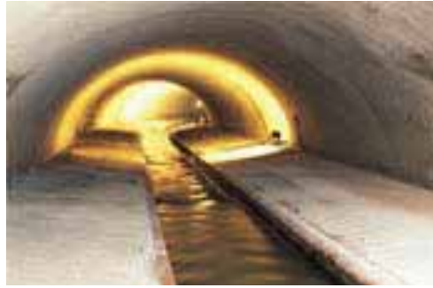
Gablenz Sewer Chemnitz, Germany. Treated areas: channel lining, walkways, creek channel; 20,000 m 2 ; products used: VANDEX UNI MORTAR 1 Z, VANDEX BB 75 Z, VANDEX PLUG, VANDEX CRS CORROSION PROTECTION AC.
