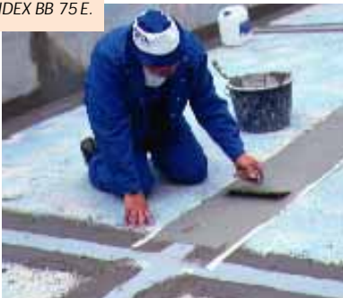
Marktöglitz open-air pool: Restoration of joints using VANDEX DILA JOINT TAPE bonded with VANDEX BB 75 E.
