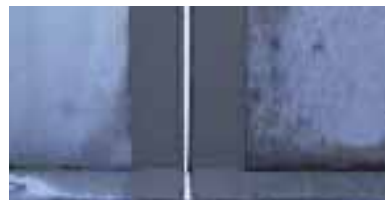
1 Apply first coat of VANDEX BB 75 E (3 kg/m 2 , 1.5 mm) at least 2 cm beyond width of VANDEX DILA JOINT TAPE.
