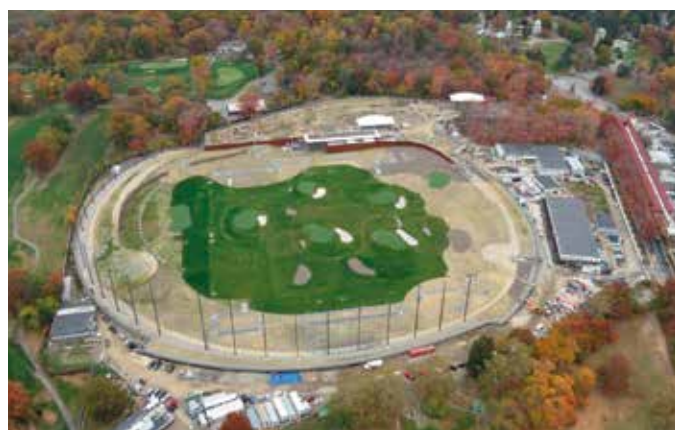
Croton Water Filtration Plant
